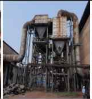
Multi cyclone sinter plant
